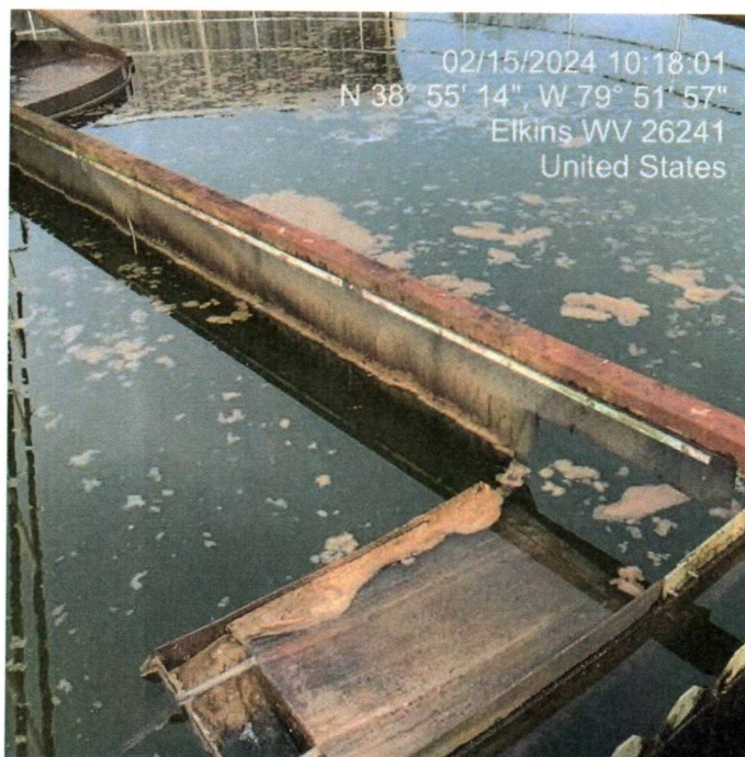
02/15/24 10:18 AM Grease balls on clarifier.
