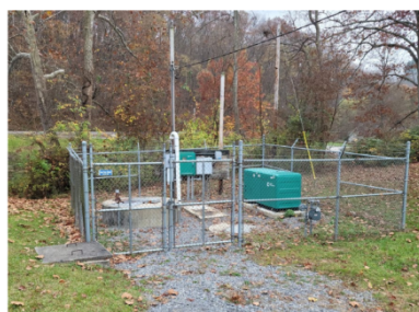
Vector Avenue Lift Station
