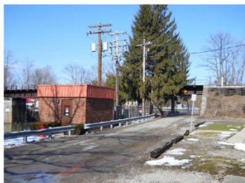
Barron Ave Lift Station
