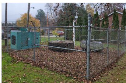
Whiteman Lift Station
