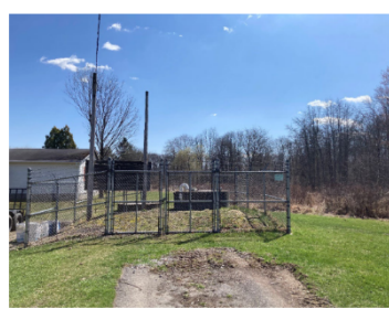
AB Andrews Lift Station
