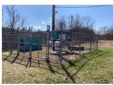
Reidboard Lift Station
