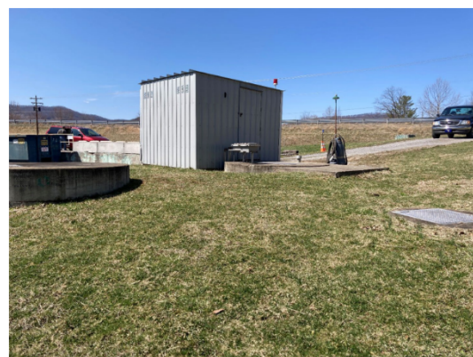
Old Plant Lift Station
